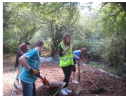
Students have prepared the ground with Mypex and spread woodchip over the surface
